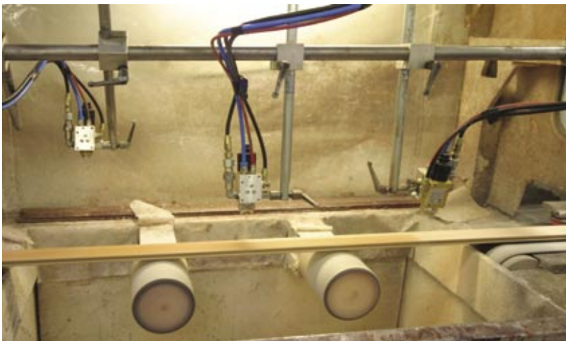
4 – The mixed-air spray-guns installed on one of the coating lines.
